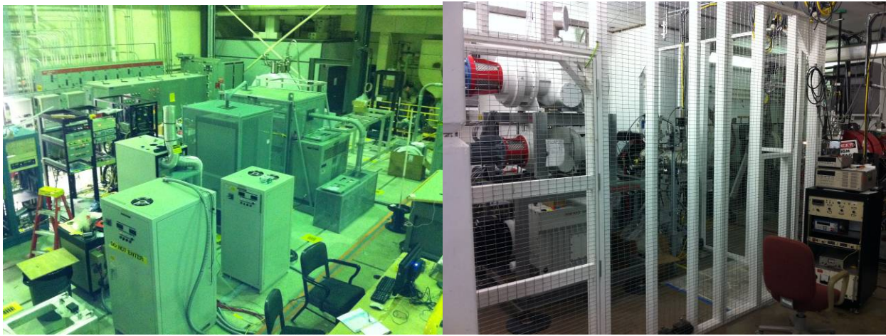
FIG. 4. Left: Equipment for the light ion guide shown positioned above the roof planks of the ion guide hall. Placement above the roof planks removes the equipment from the high radiation environment of the ion guide hall. Right: The three tier roots blower system and high voltage safety cage for the light ion guide system shown completed in the ion guide cave.
