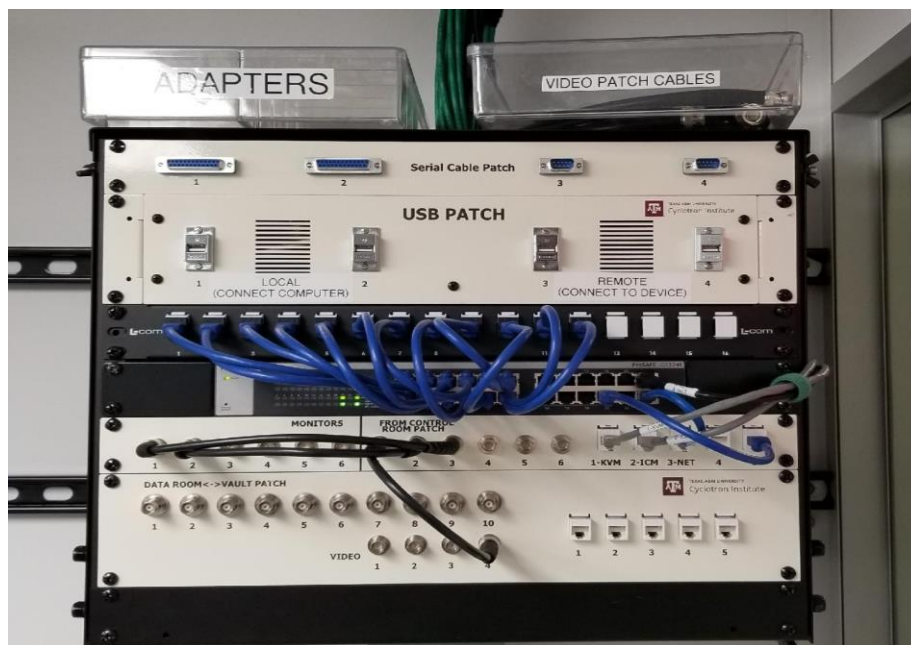
FIG. 1. Network, computer, and data patch for communication between K150 Data Room, K150 Radiation Effects Beamline, and the Control Room.
