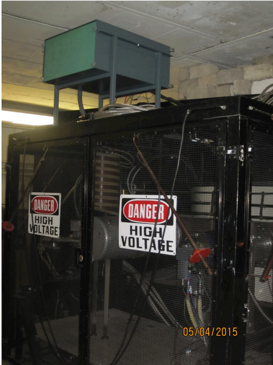
FIG. 1. The deflector power supply was relocated closer to the deflector above of the deflector cage. The supply is shielded from neutrons inside a box with 3 layers of 1" borated polyethylene panels.
